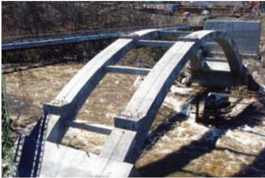
Above A cap beam is aligned for the Route 52 bridge over the Wallkill River in Walden, N.Y.
