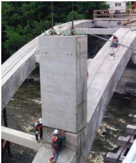
Above The column section is erected for the Route 52 bridge over the Wallkill River in Walden, N.Y. Photo courtesy of Rohit Dagli.
